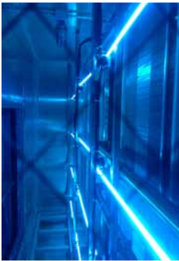
Typical large HVAC System with UV-C fixtures
