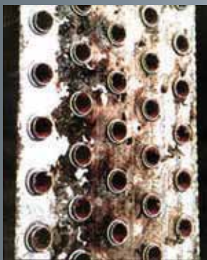
Cut Coil Shows Impacted Mold and Dirt Increased Pressure Drop Less Airflow Reduced Heat Transfer
